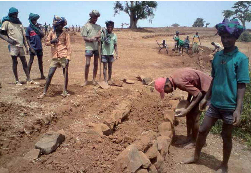
Building terraces is a climate change adaptation strategy of the local population in Ethiopia.
